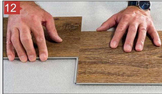
STEP 12: Disassembling the short side Finished? Remove spacers and cover gaps with a trim.
